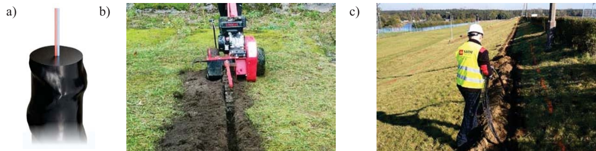
Fig. 5. Application of EpsilonGraph in earthdam: a) sensor visualisation; b) trench along the entire length of the head dam; c) installation of the sensor within the trench.
