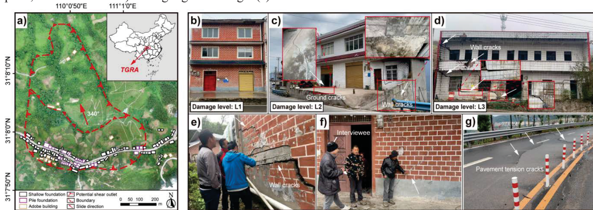
Fig.1 Landslide I and in-site survey: (a) location;(b-d) typical buildings with different damage levels; (e,f) crack patterns of brick-concrete buildings; and (g) pavement tension cracks.
