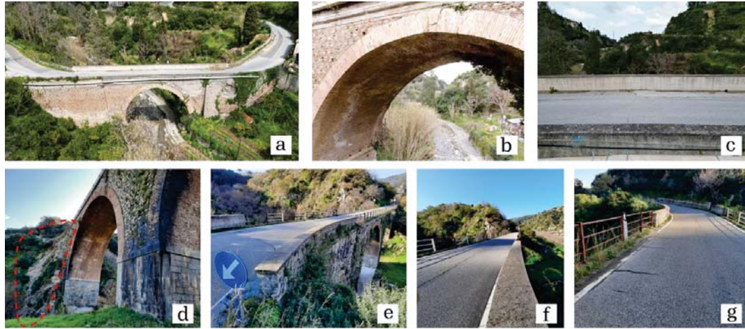
Fig. 3. Evidence from the second case study: a) overview of the structure with evidence of significant repairs; b) detail of the arch showing cracks on the arch barrel and intrados; c) cracks on the asphalt pavement. Evidence from the third case study: d) view of the abutment with signs of instability and masonry damage; e-f-g) cracks on the road surface and parapet walls.
