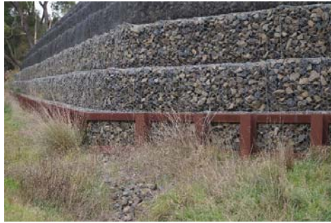
Figure 1. Slope site reinforced by the integrated method that comprises the pile retaining wall with GF-GR-RW
