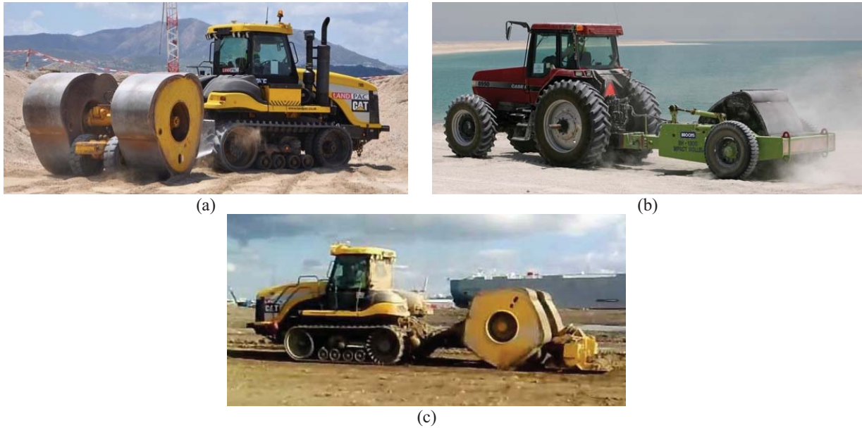
Figure 6. Rolling dynamic compaction modules: (a) 3-sided (Landpac); (b) 4-sided (Broons); (c) 5-sided (Landpac).
