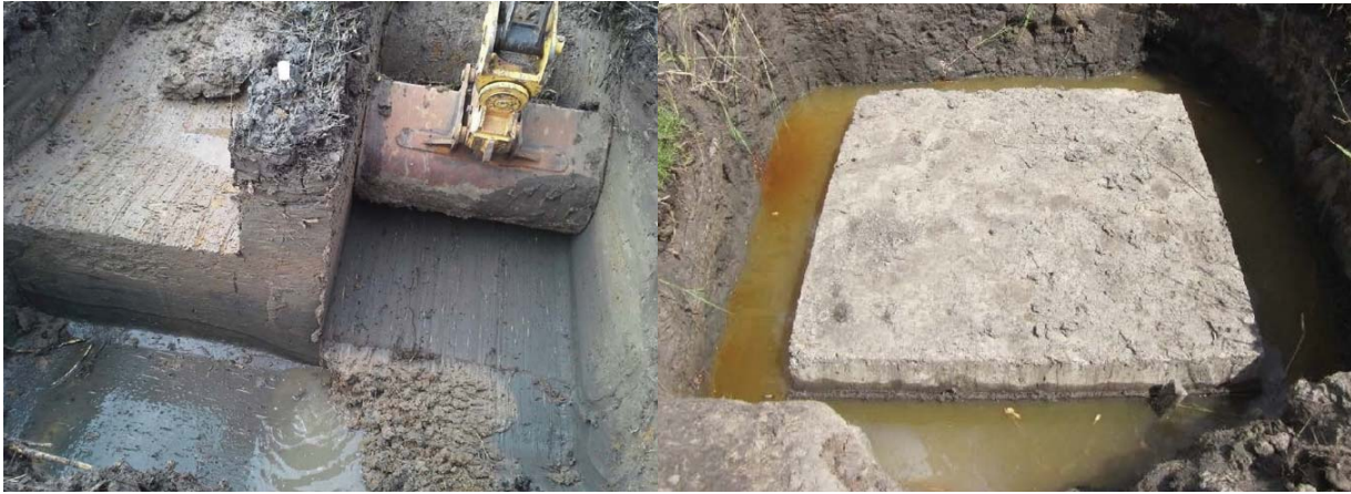
Figure 13. Careful excavation for 1 m square pad footing on soft marine clay and the cast footing prior to test
