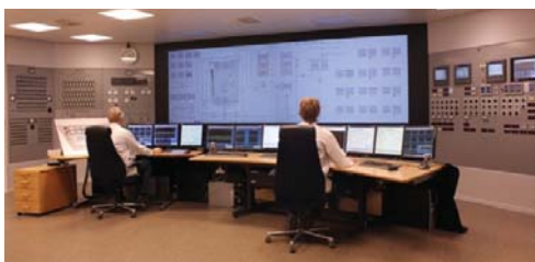
Fig. 3. HBWR control room environment.
