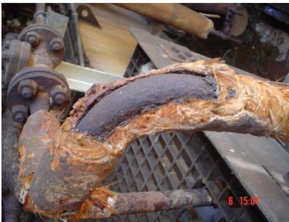
Figure 8.13. Corrosion inside an insulation due to high temperature and possible intrusion of water inside the insulation. (Courtesy: Balaji.)
