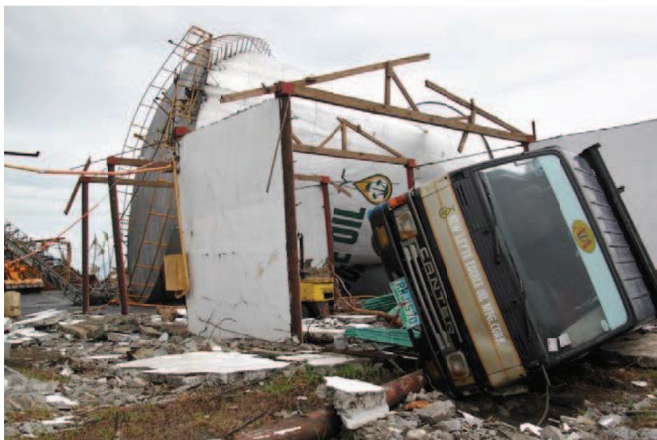
Figure 4 Damaged oil tanks in Tacloban (phot credit: UNDAC/D.Bruhn).
