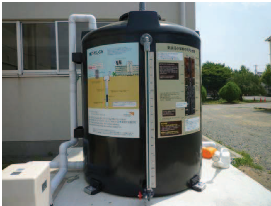
Figure 3 The well with solar panel of Kesennuma Elementary School.
