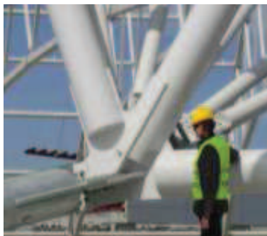
Figure 1. Abrupt connection of tubes
