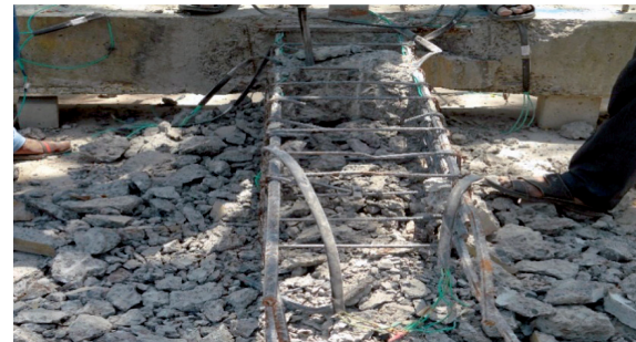
Fig. 5 Exposed reinforcements of beam
